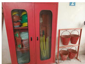
Fire fighting equipments.jpg
