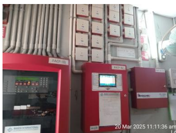
Fire alarm control panel.jpg
