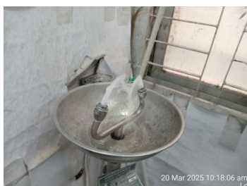
Eye wash station.jpg
