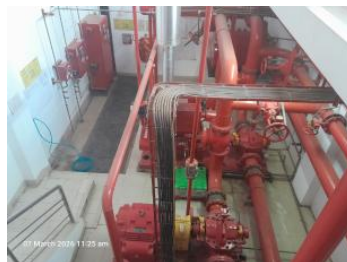
Fire pump room.jpg
