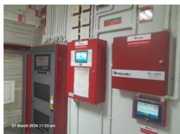
Fire control panel.jpg
